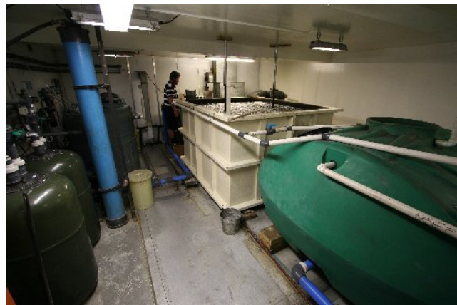
Anton at work in the waste-water processing room
